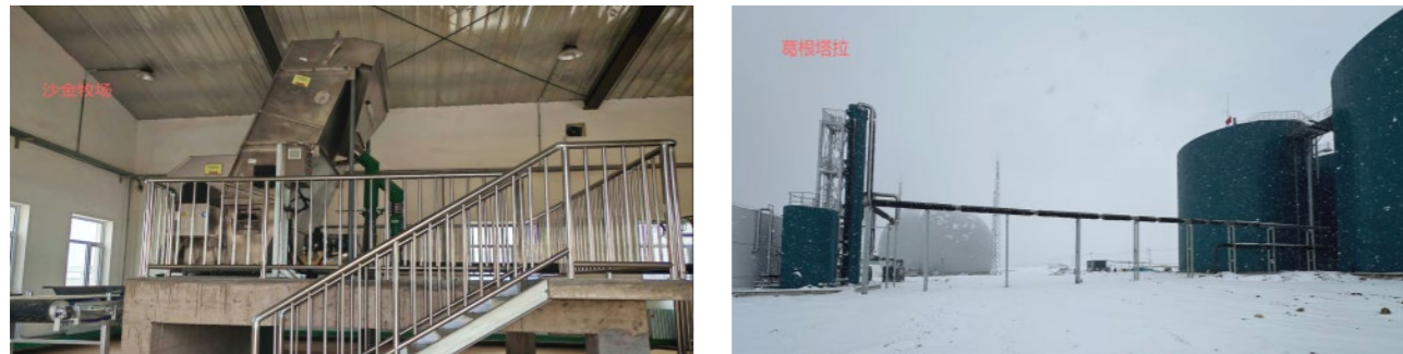
Farm Manure Treatment Facilities
